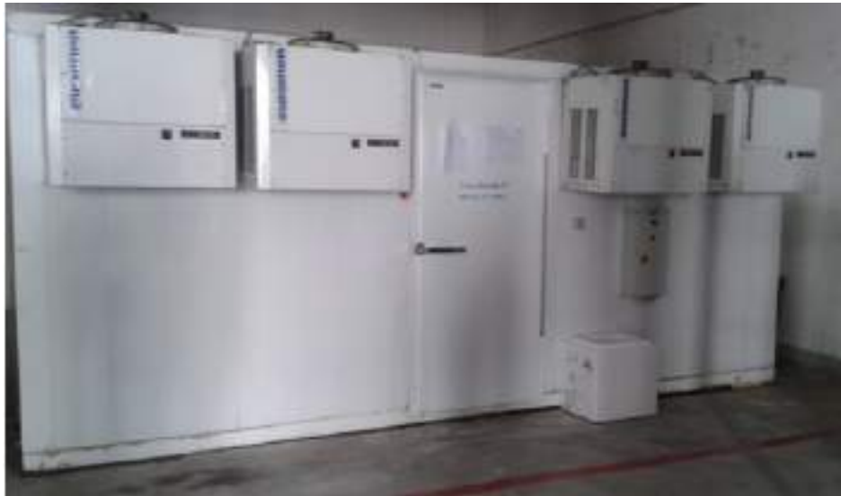
Figure 20. Freezer Room 50 m 3 Capacity at Store
