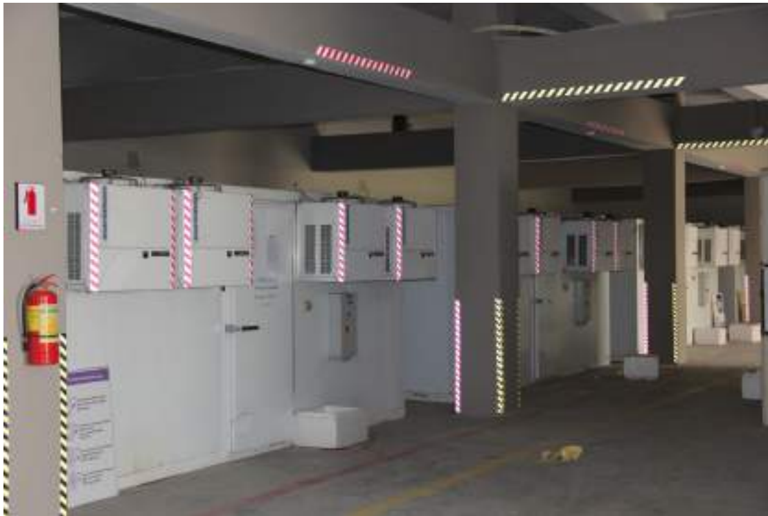
Figure 19. Cold Room 50 m 3 Capacity at Store
